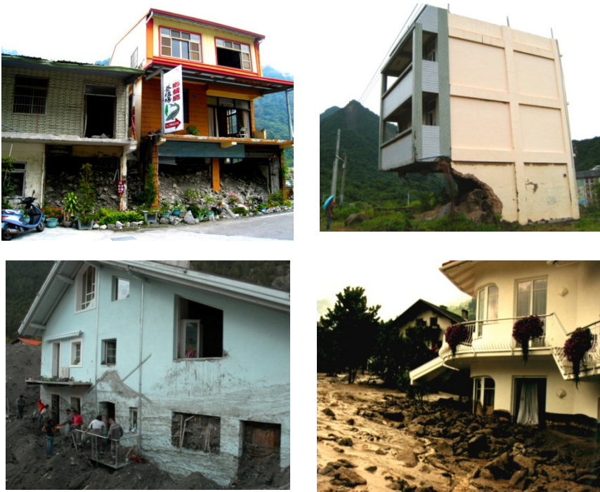
Figure 3: Typical damage patterns for buildings affected by torrent processes in Taiwan (top) and Austria (bottom). Upper left: Songhe community, Taiwan, August 2004, upper right: Min-Zu community, Taiwan, August 2009, lower left: Pfunds community, Austria, August 2005, lower right: Wartschensiedlung village, August 1997. Credits: upper left and right: S. Fuchs, lower left: GBL 6.2, lower right: anonymous.
